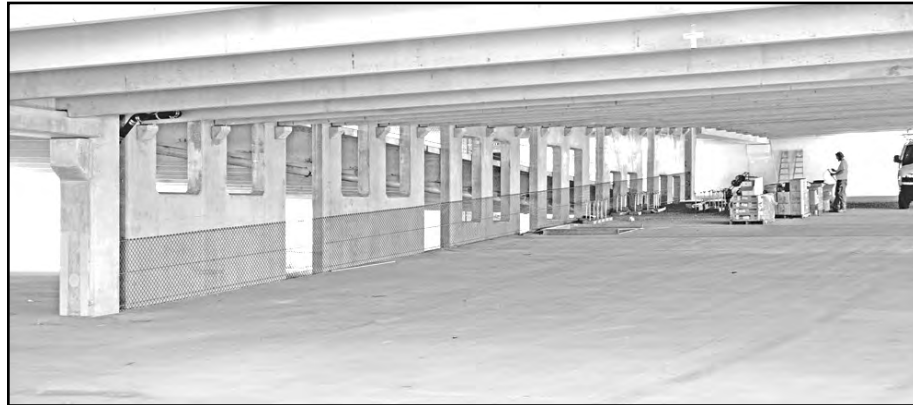
The massive three-story parking garage at Rosie's is ADA accessible and features an elevator.
