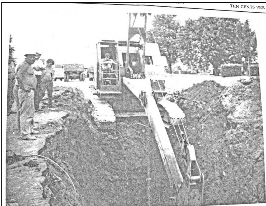
In July 1972, Town of Vinton workers were busy repairing an 8-inch sewer main buried some 23 feet deep on Blandford Avenue. The main and lateral lines had been causing problems for 5 years.
