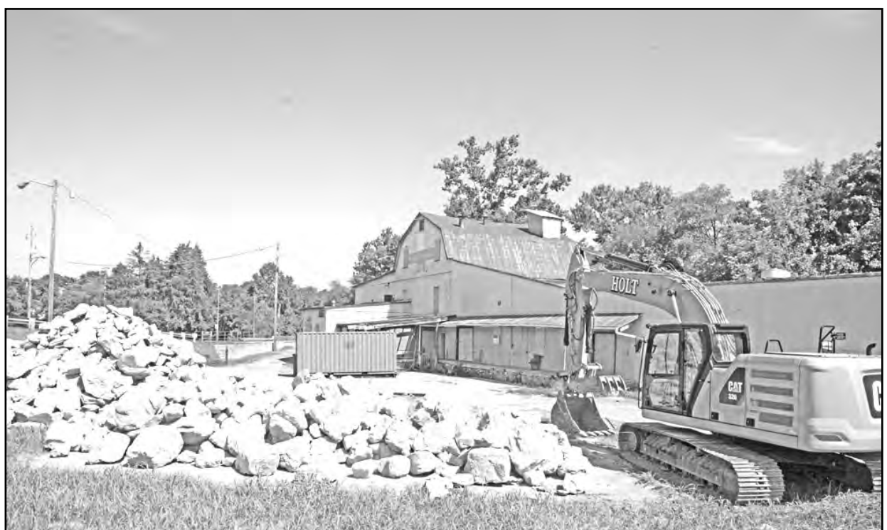
PHOTO BY DEBBIE ADAMS A giant pile of boulders at the historic Gish Mill site will be used for stream bank stabilization along Glade Creek.
