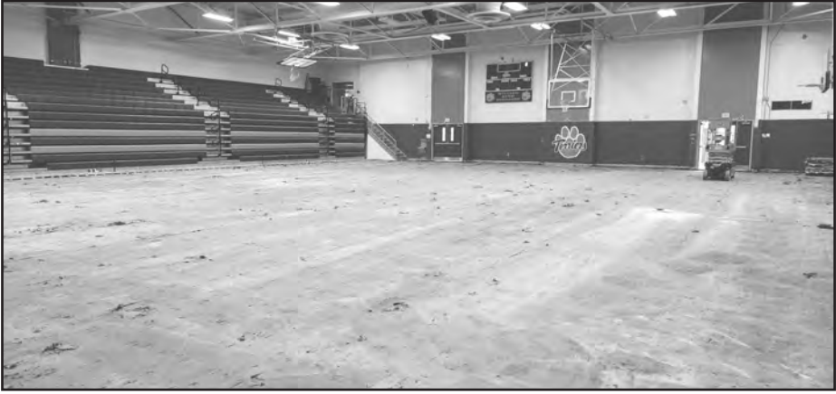
Demolition of the main gymnasium floor has been completed at WBHS, except under the bleachers.
