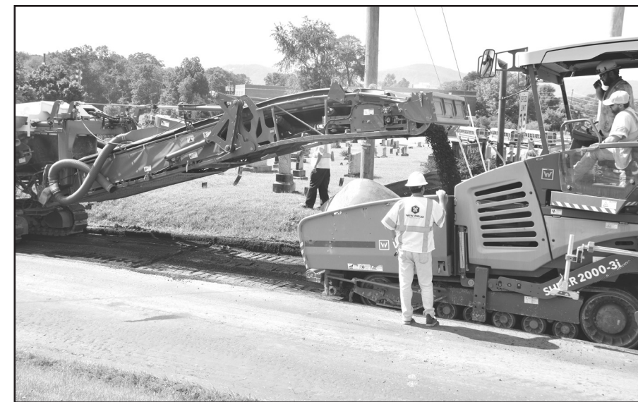
In the FDR process, existing pavement is pulverized and mixed with cement powder and water to form a stabilized base for the roadway.
