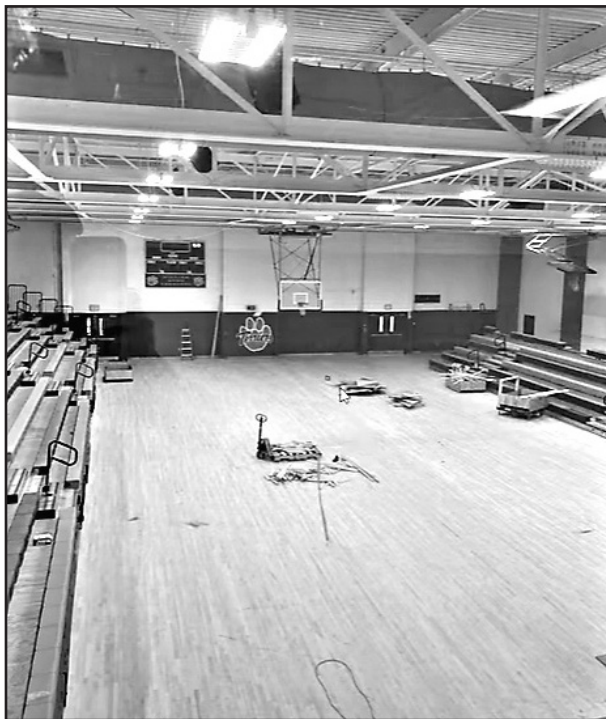
The wood has been installed for the gymnasium floor with completion expected by August 31.
