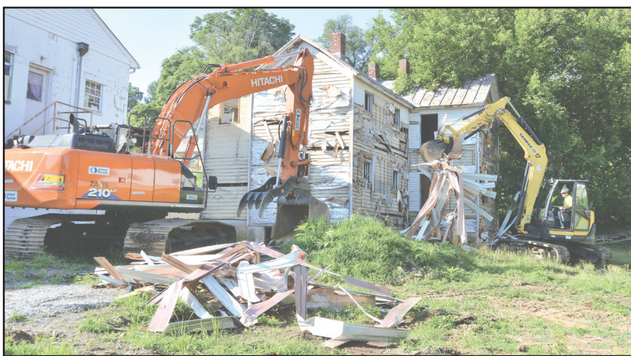
Demolition by Public Works employees Kenny Sledd, Billy Robb, and Banks Bradford on July 11.
