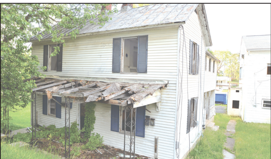
The 1920s house on Cleveland was demolished by Vinton Public Works employees as part of the Cleveland Mart Redevelopment Project.
