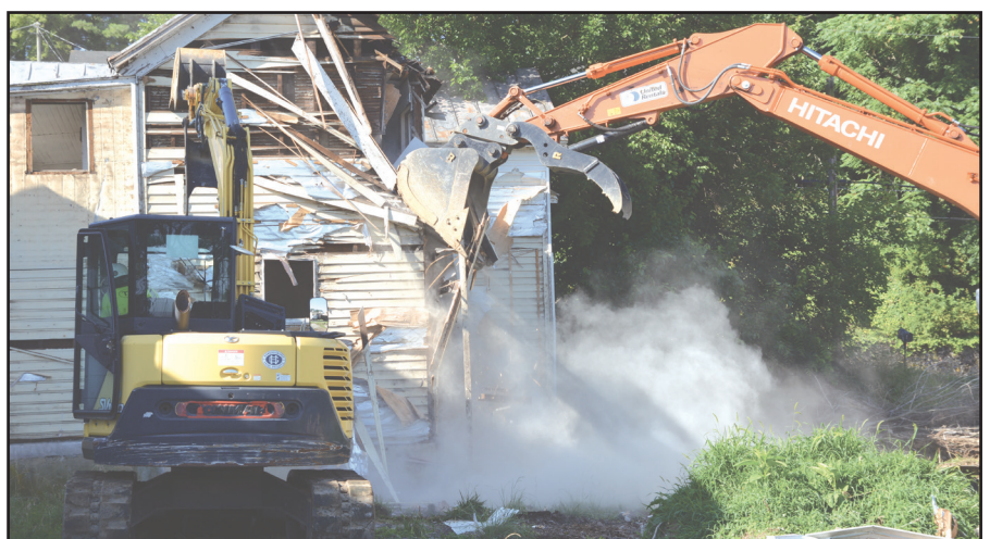
PHOTO BY DEBBIE ADAMS Demolition for the Cleveland Mart Redevelopment Project continued on July 11 with removal of a house next door to the Cleveland Mart. The store itself will be renovated, not removed.
