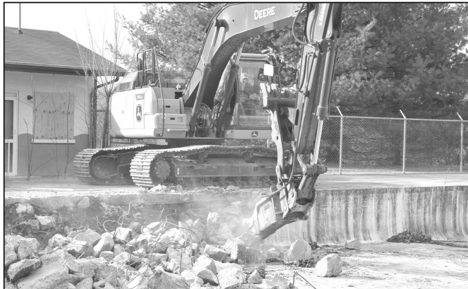
Once the pool is demolished, the space will be filled in, in part, with the concrete from the pool.
