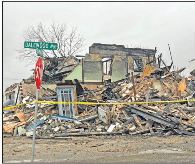
The former Givens Books building at 1641 East Main Street caught fire on the night of Tuesday, Dec. 6.
