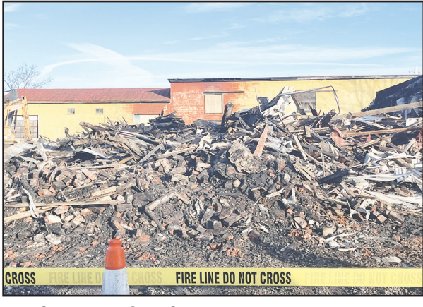
The Salem Fire & EMS Department responded to a fire at 17 7th Street at approximately 2:30 a.m. Monday morning.
