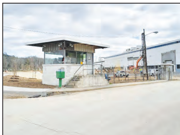
Contractors deliver supplies for an addition to the former Salem GE facility where a $32-million Volvo-related production facility will be.
