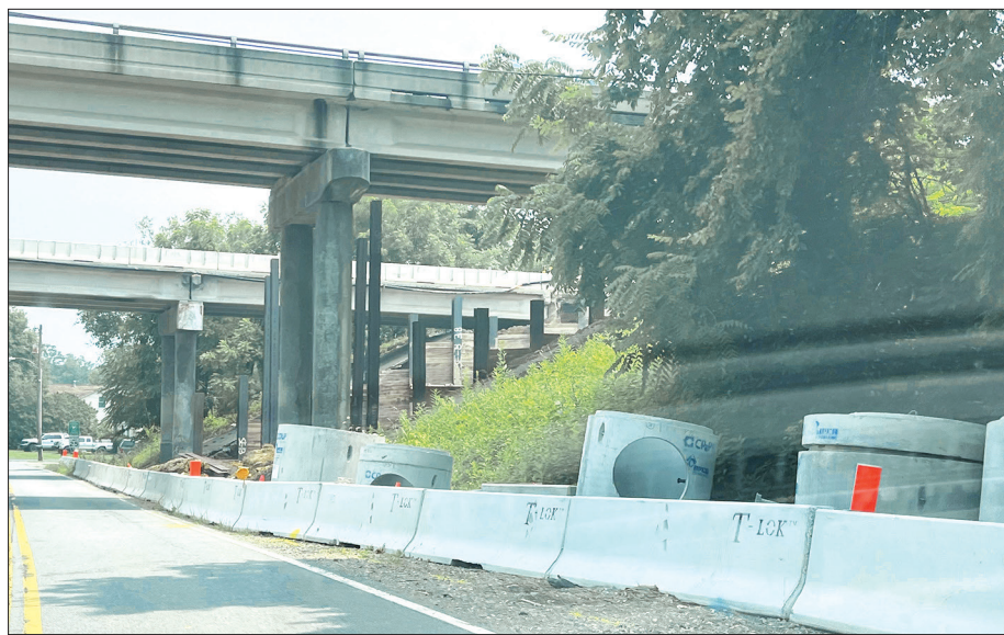
The repair work that was done is pictured from Goodwin Avenue on Monday.
