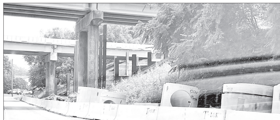
Flaggers were periodically controlling traffic on Goodwin Avenue and Academy Street beneath the bridges during the repairs.
