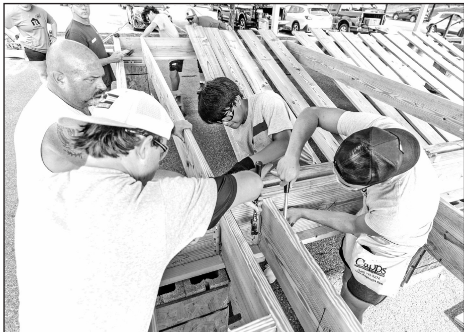
Students, volunteers and Habitat for Humanity staff work together on the R House.
