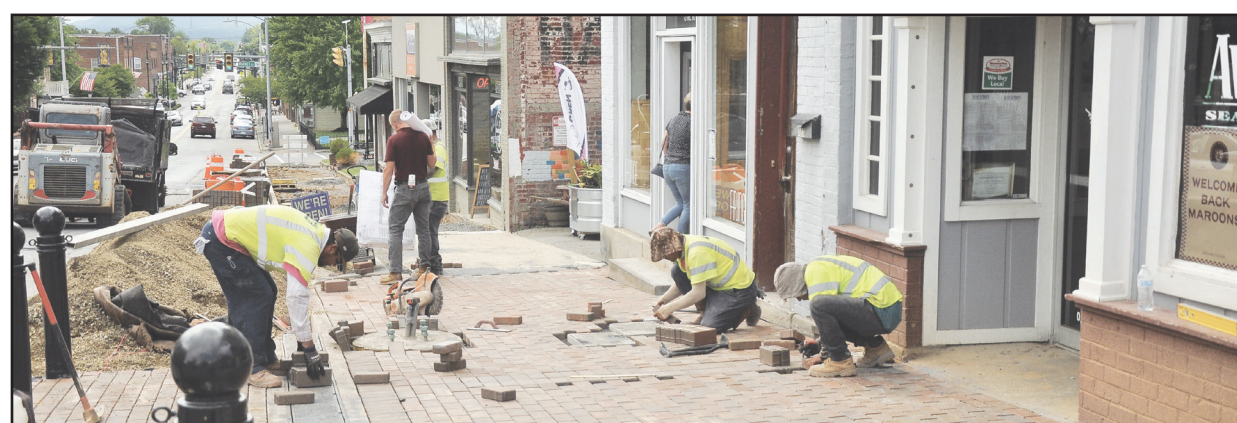
Workers lay bricks for the new sidewalk on Main Street last week.
