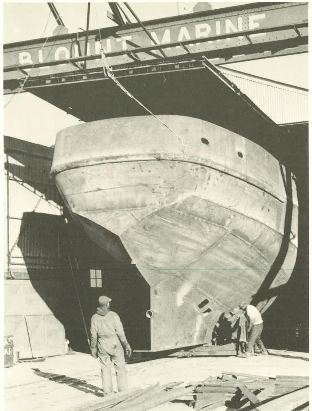
Stern view of dragger CAP'N BILL III emerging from main construction shed at Blount Marine.
