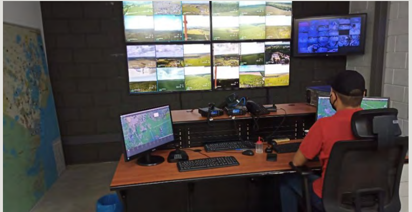
18 towers equipped with fixed and mobile cameras at FBU-ES
