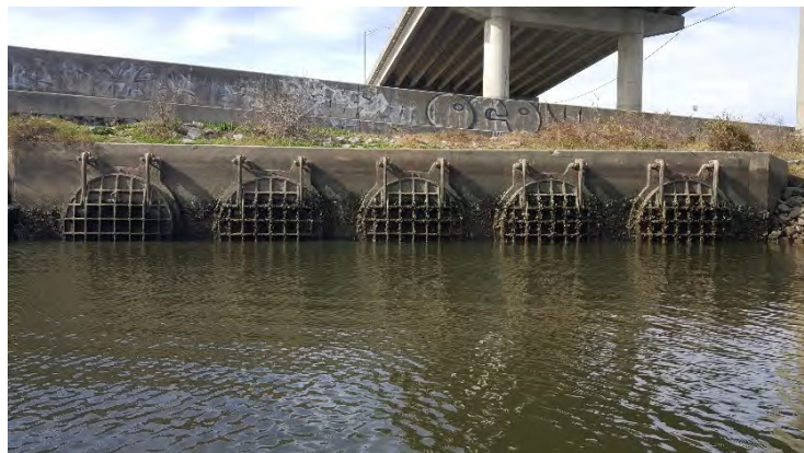
Tidal gate at Virginia Avenue. (Photo by Three Oaks Engineering)
