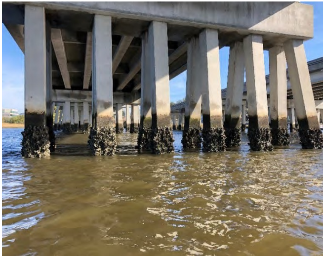
Oysters on existing bridge structures in the Ashley River. (Photo by Three Oaks Engineering)
