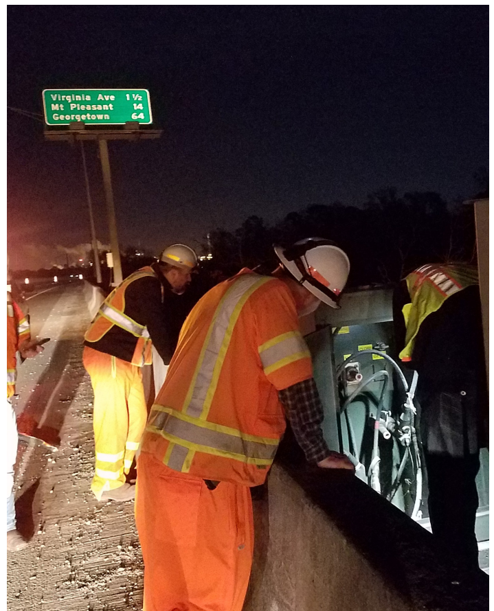
Nighttime inspections were conducted on the Don Holt Bridge's existing electrical systems.
