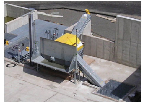
Concrete Pump Washout "PDC" module
