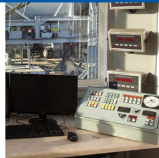
RC3 Batch Automation Controls
