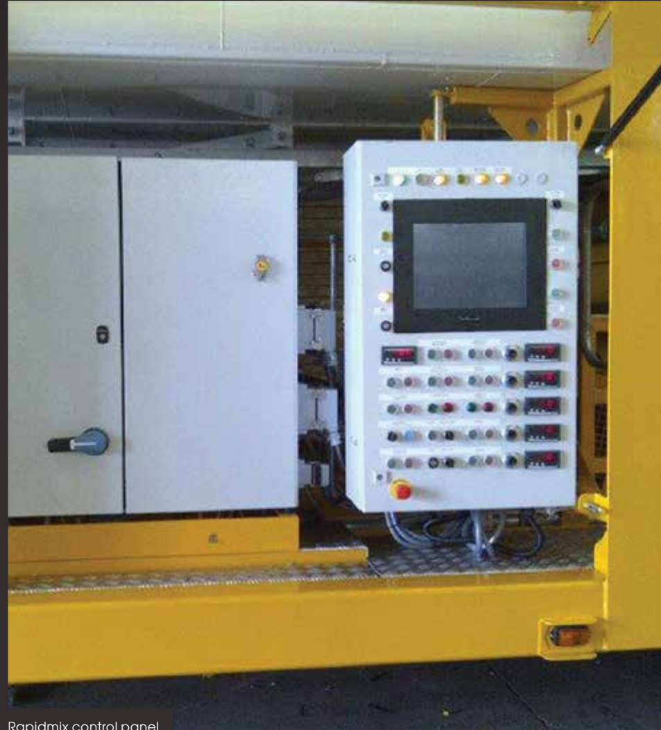
Rapidmix control panel
