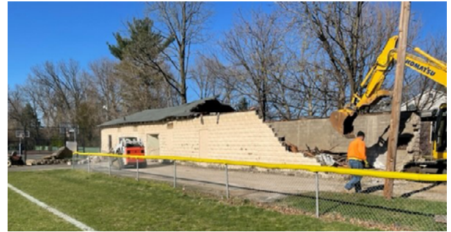
This week the field house at Tamblin Field was removed in the first step of phased-in improvements to the Tamblin Field overhaul. Bids for pickleball and basketball courts are currently being reviewed.
