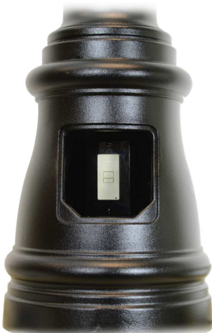
15A Ground Fault Breaker, in base (GFB)
