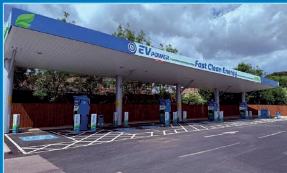
EV Charging Hub
