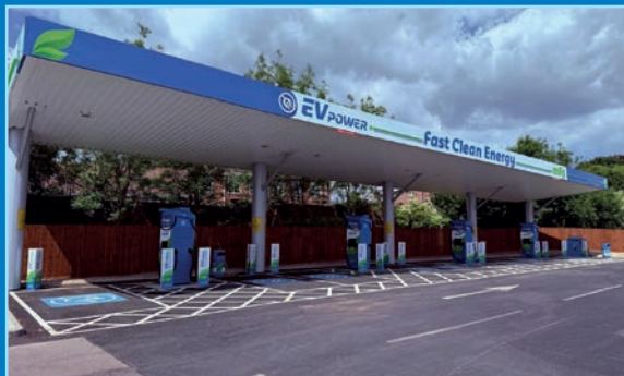
EV Charging Hub
