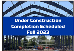
Under Construction Completion Scheduled Fall 2023 Jim Green Indoor Track & Field Center Sports Center Drive
