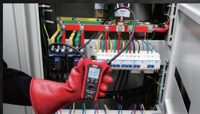
Bus bar current test
