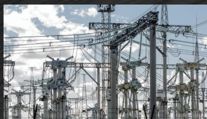
Power distribution station
