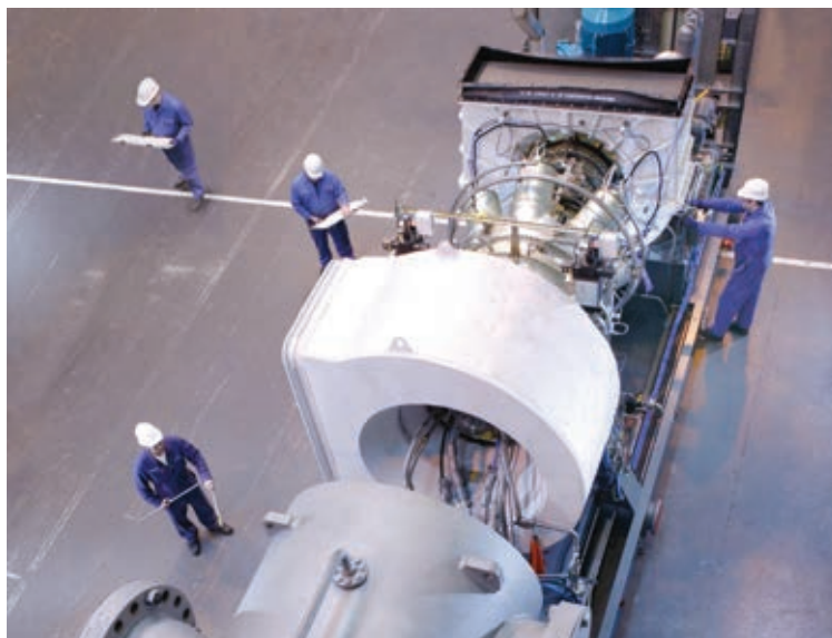
Photo courtesy of Siemens
