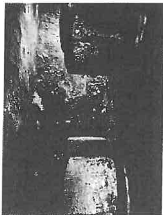
Leak at 36" Flange on 42" Tapping Sleeve
