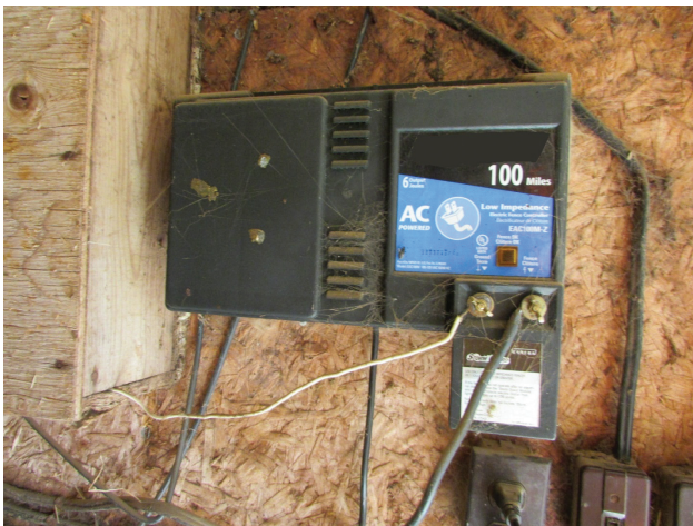
Picture 16: Example of an electrical fence energizer
