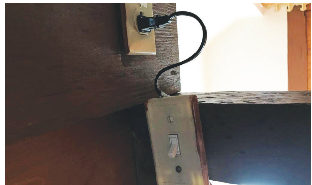
Picture 12: Example of an unapproved electrical installation of a light switch
