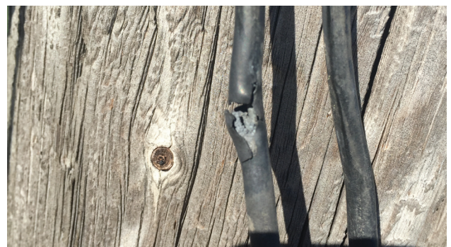
Picture 2: Example of an LDC grounding conductor on the pole that has been damaged
