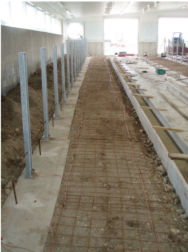
Picture 3: Example of metallic mesh installation used to create equipotential.
