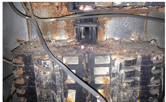
Picture 8: Example of a deteriorated electrical panel
