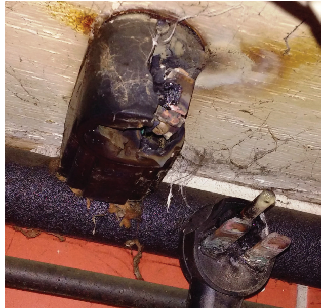
Picture 14: Example of receptacle damaged from corrosion and arcing
