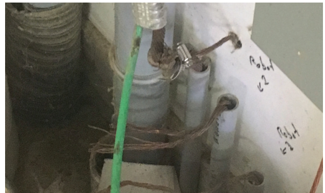
Picture 1: Example of a disconnected bond wire
