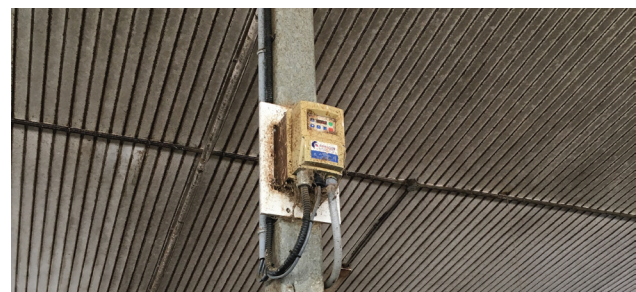
Picture 15: Example of a VFD
