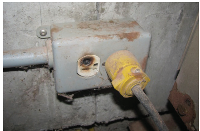
Picture 9: Example of a damaged receptacle
