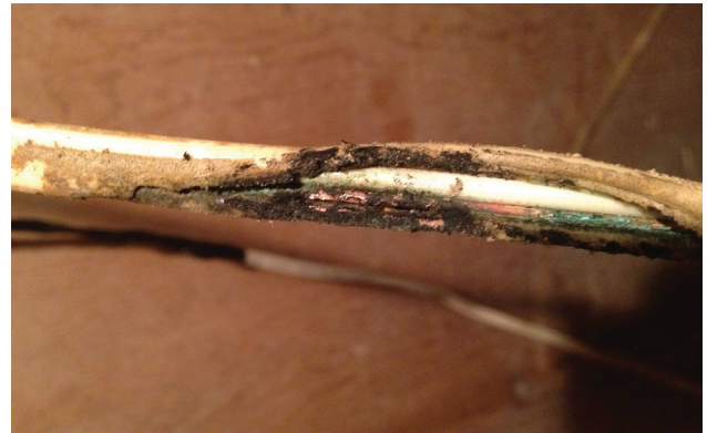
Picture 4: Example of conductor insulation damage.
