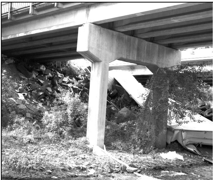
Debris is scattered under the westbound lanes of I-90 at the Cedar Creek bridge, and the rear of the semi appears flattened from the impact. The vehicle landed on the east side of the creek between the two bridges. (Photo by Mary Jo Berry.)
