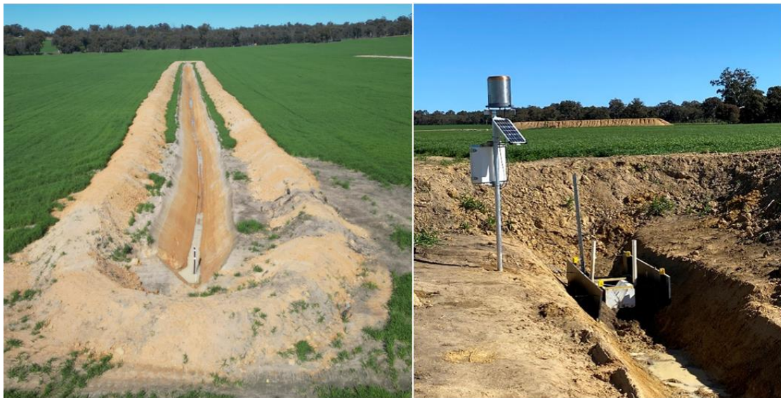
Figure 13. Left: South's site open V subsurface drainage system. Right: Ground-level image of the 11-inch Parshall flume and rain gauge monitoring equipment.
