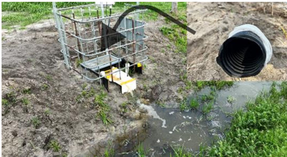
Figure 10. Photograph of Ashton's site 11-inch Parshall flume outlet with the insert photo showing the style of agricultural pipe used
