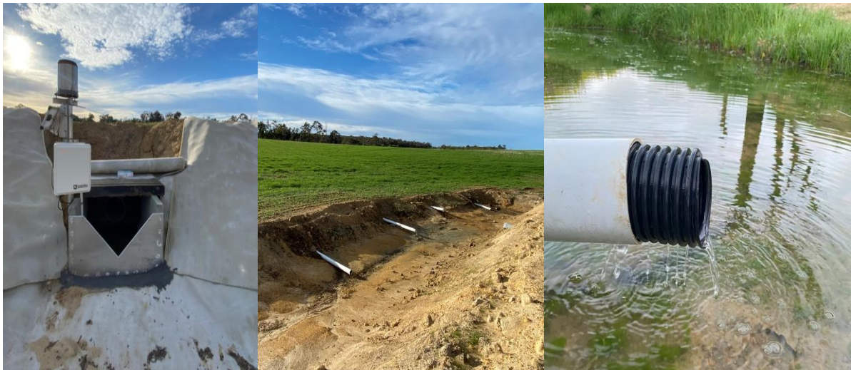
Figure 12. V-notch weir setup at Webbs (left), Four tile drains ending at the sump above the dam (centre), Tile drain running on 20/8/2025 (right).
