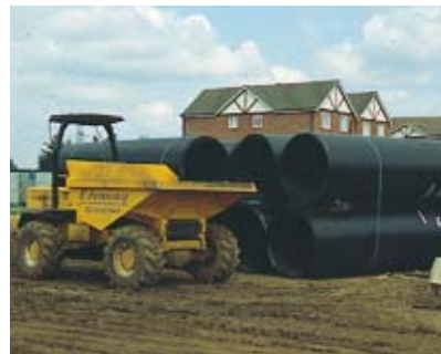
Rainwater storage tanks
