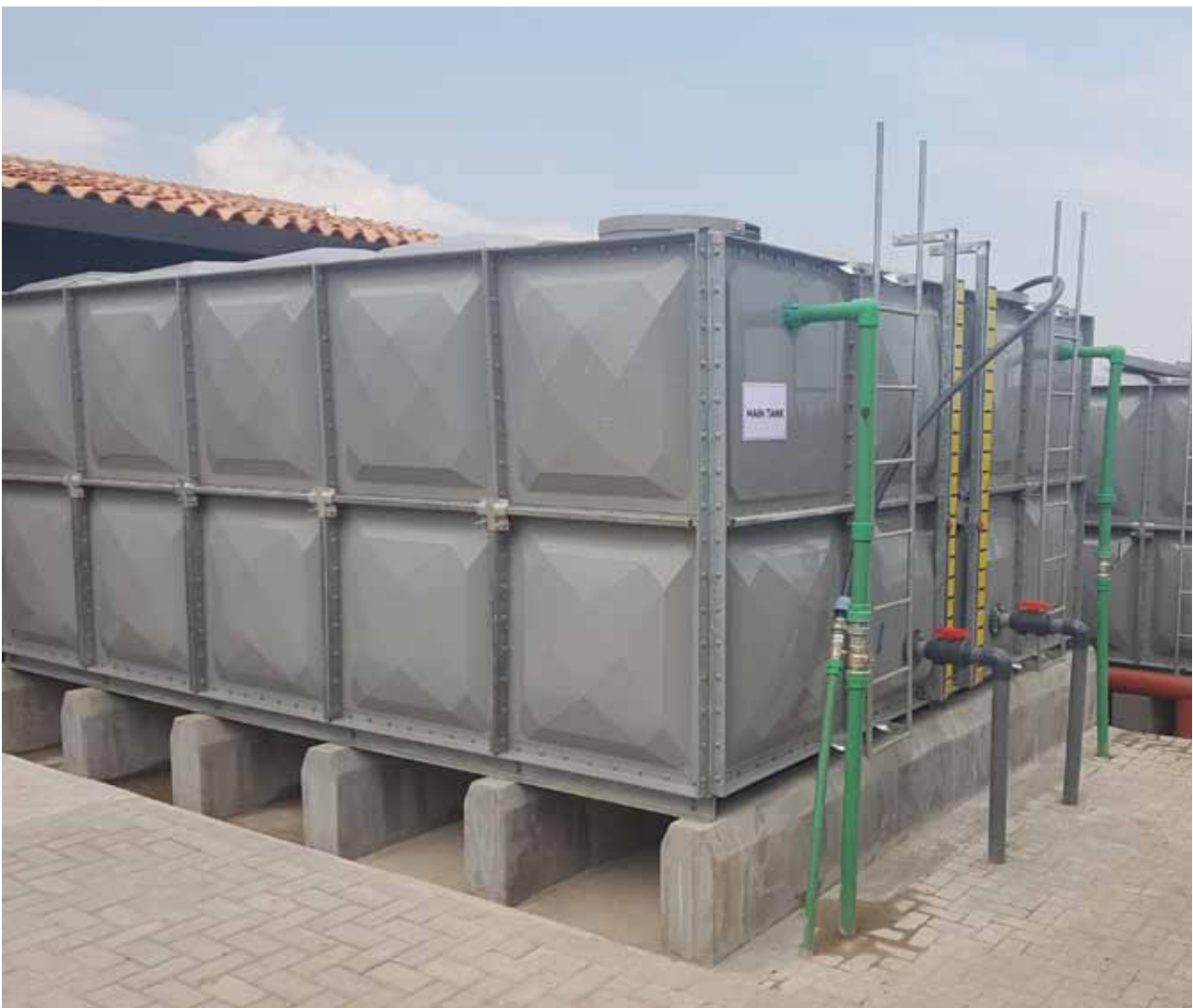
Potable water reservoir at installation
