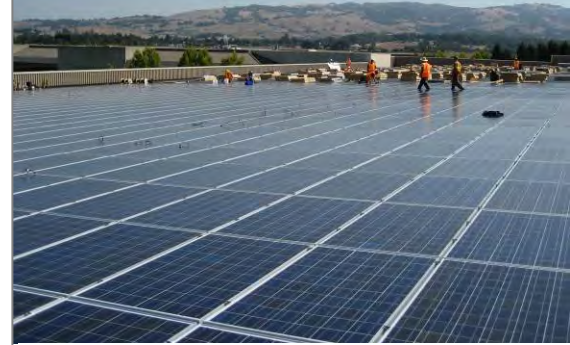
Workers install the solar power plant at Sonoma Mountain Village. The $7.5million plant generates 1.14 megawatts – enough to power 1,000 homes.
