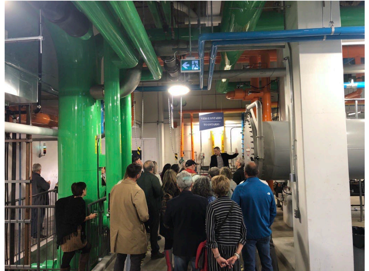
Tour of the ZCU Central Plant © Zibi
