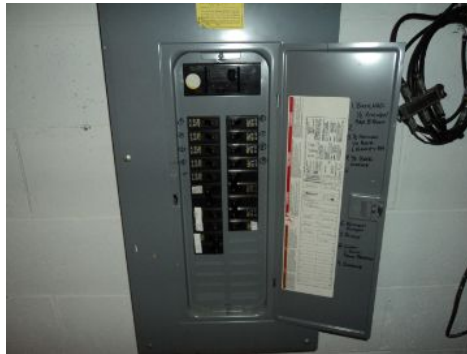
Main panel - Location in the garage.
