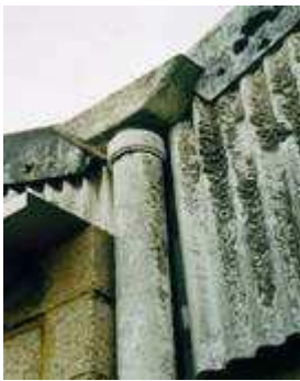
Asbestos cement drainpipe and cladding
