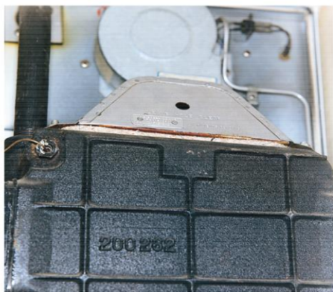
Inside Gas boiler Asbestos seal
