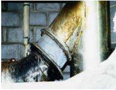
Flexible asbestos duct connector (Gaiter)
