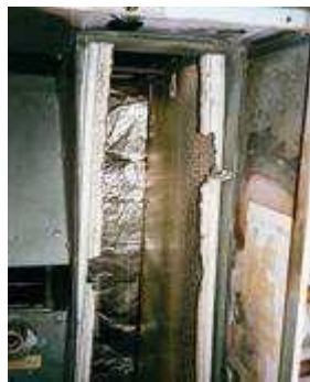
Asbestos paper lining
