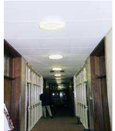
Asbestos ceiling tiles
