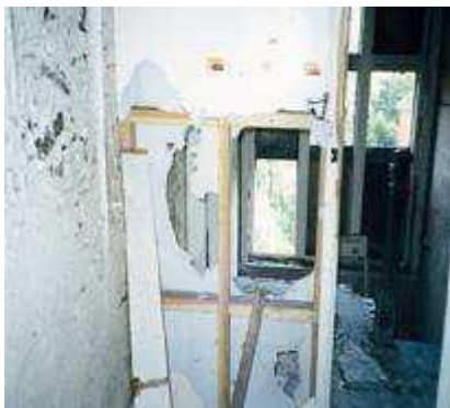
Badly damaged AIB panel
