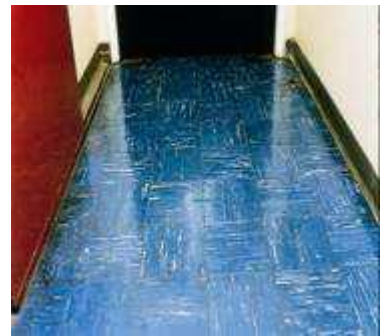
Asbestos-containing floor tiles
