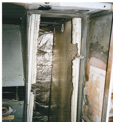
Warm air heater Asbestos paper
