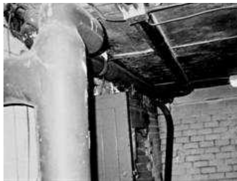
Asbestos debris on stripped pipe-work
