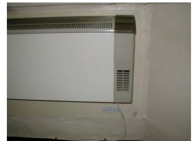
Asbestos panel behind heater and in heater
