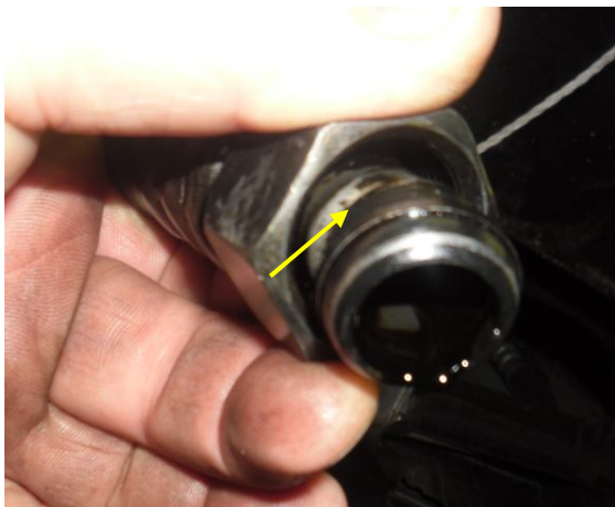
Oil leakage occurred from this joint
