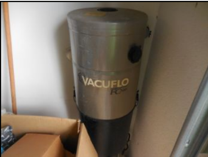
Central vacuum was working.
