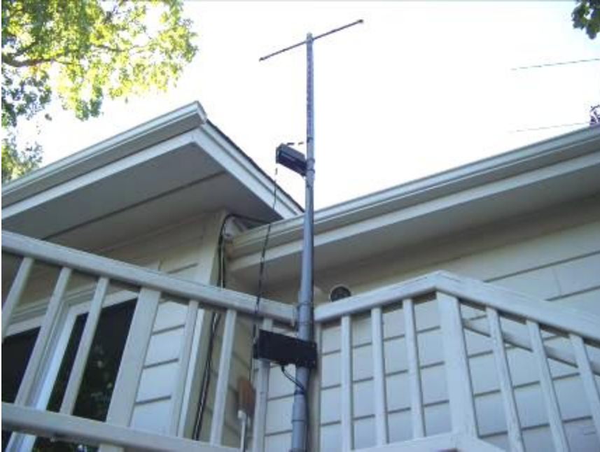
Connection of the loops to the matching support structure A 144/440 MHz vertical and 6 meter beam with its radials is in the back ground.
