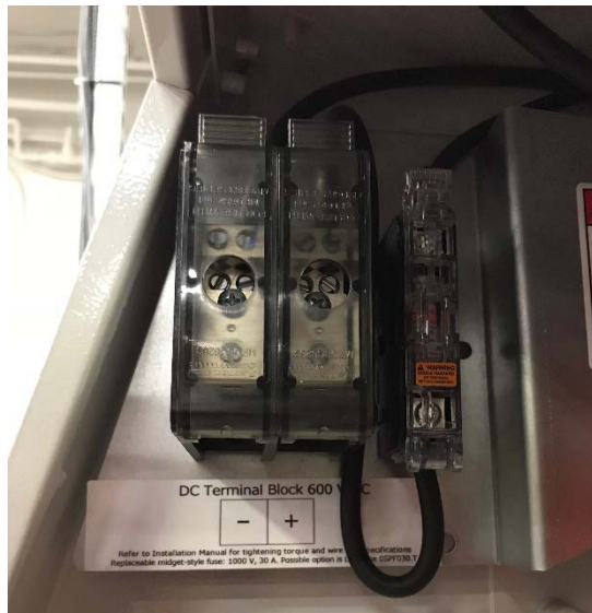
Figure 10 – Main HVDC landing Distribution Block.
