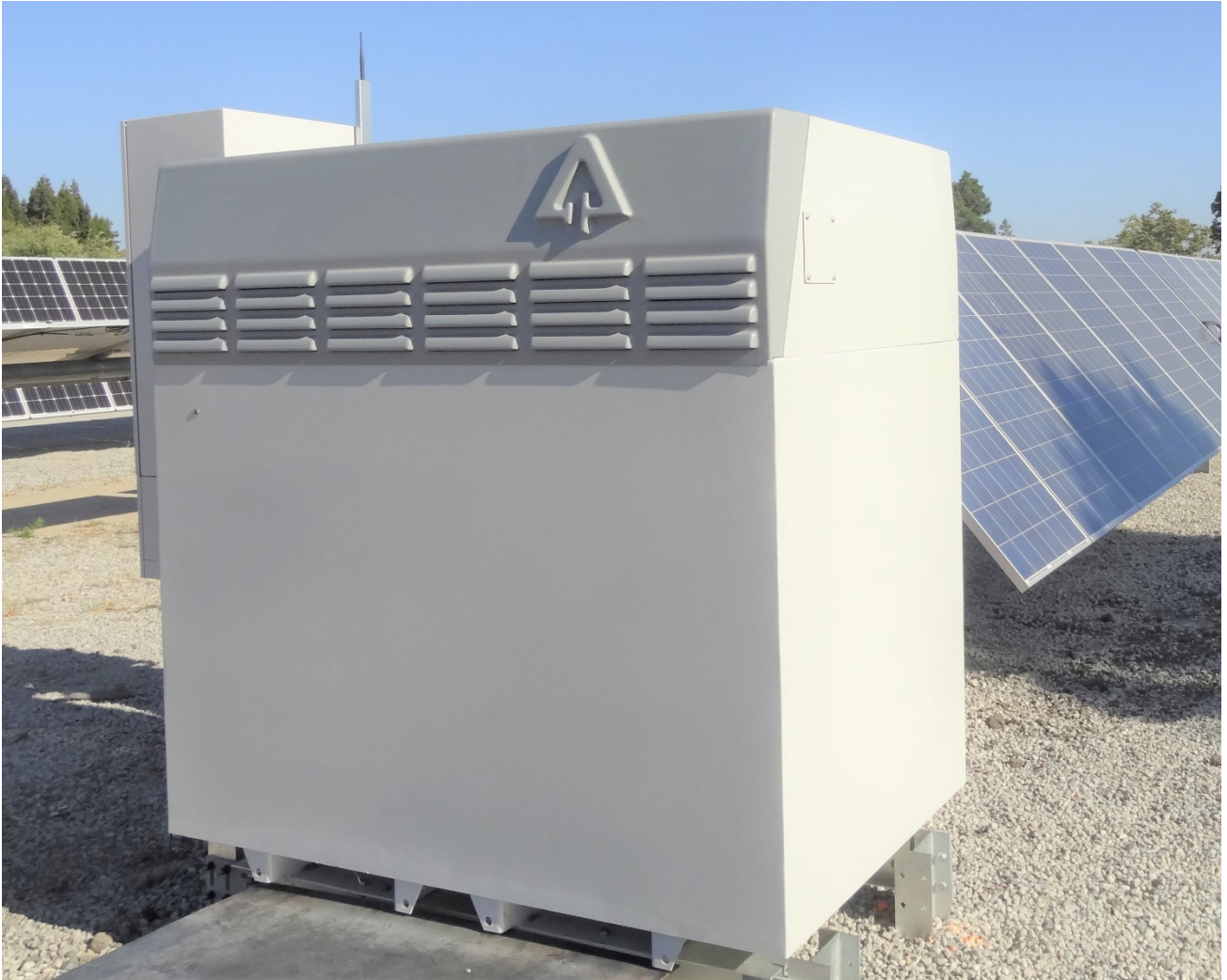
Figure 1 – AFB2 Vanadium Flow Battery.
