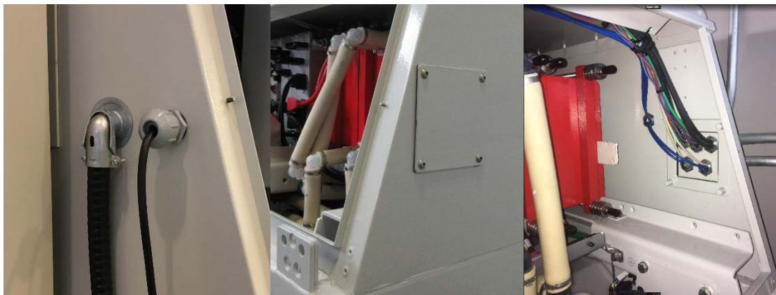
Figure 8 – Knockout locations on the AFB2 battery. 1-1/4" and 3/4" knockouts shown on the left, and panel allocated on the right shown in the middle for any required pass throughs, and the same panel modified to connect with additional batteries shown on the right.
