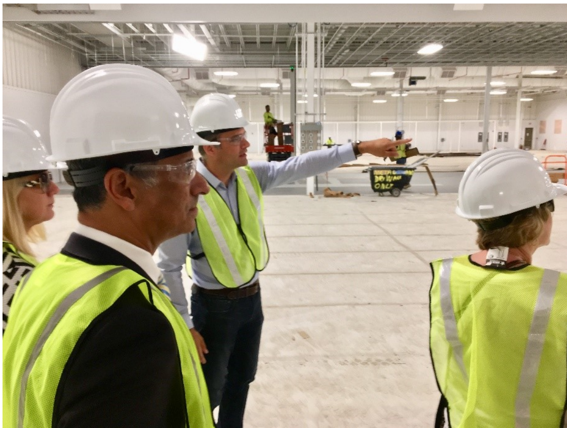
Kai Schmidt, Airbus OneWeb Satellite's HR Director, and Consortium Chairman explains the production hall layout to Representative Asencio at OneWeb's new manufacturing facility at the Kennedy Space Center's Exploration Park
