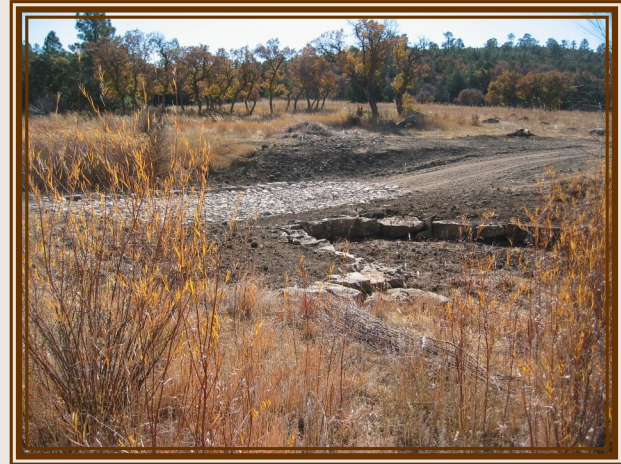
Repaired road crossing along a streambed on private land in NM (USFWS/NWTF project) (Scott Lerich - NWTF)
