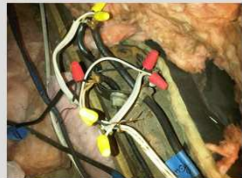
Open joints in an attic space
