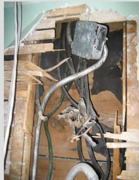
Open joints that were hidden inside a wall
