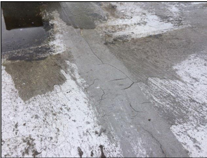
1. Surface cracks, splitting
