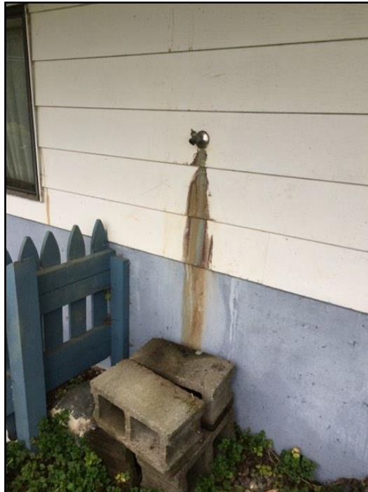
42. Leak or drip
