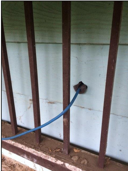
33. Exposed on walls or ceilings
