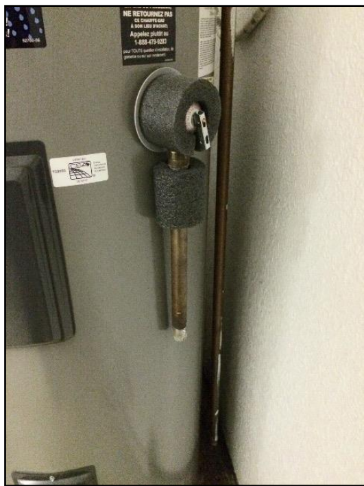
41. Discharge tube too short
