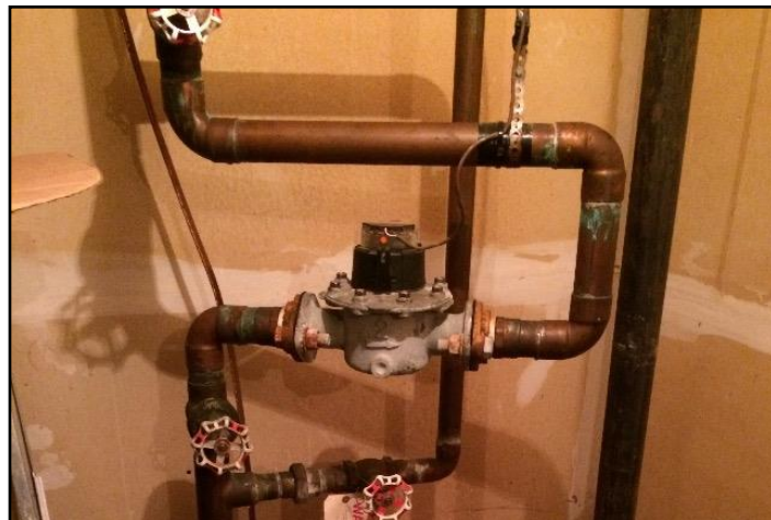
39. Required due to high supply water pressure
