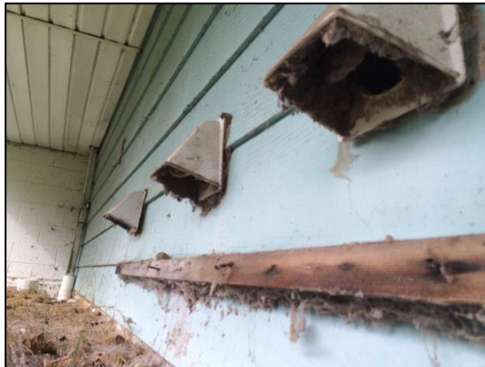
46. Screen on vent termination
