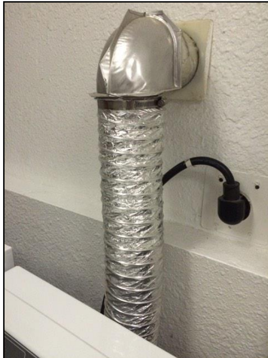
45. Dryer vent material not smooth wall
