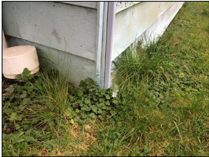
28. Siding too close to grade
