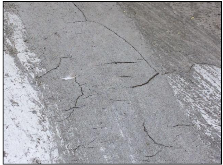
2. Surface cracks, splitting
