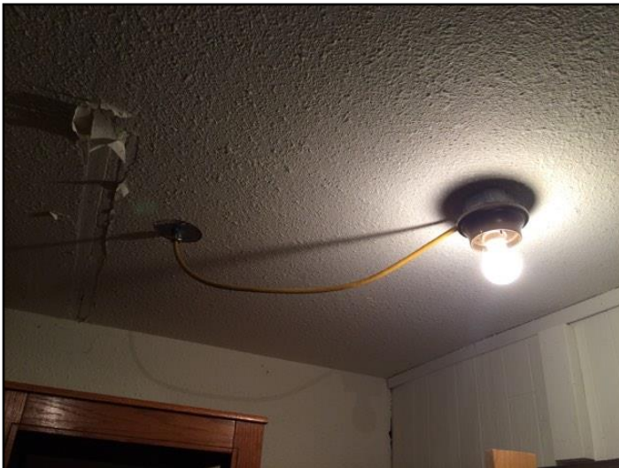
35. Exposed on walls or ceilings
