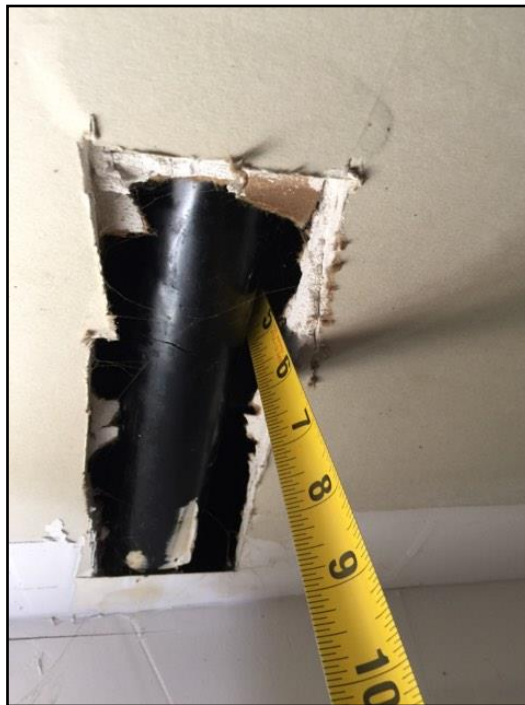
39. Floor joists undersized
