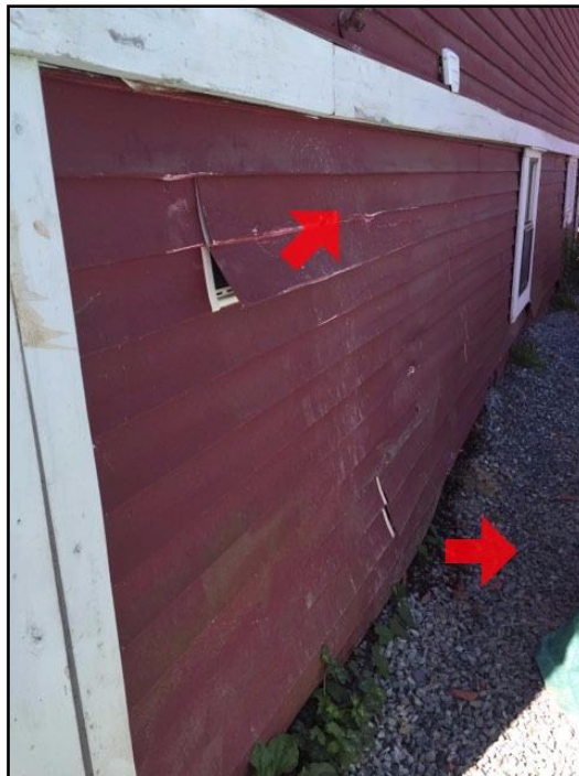
22. Vinyl siding buckling and pulling away
