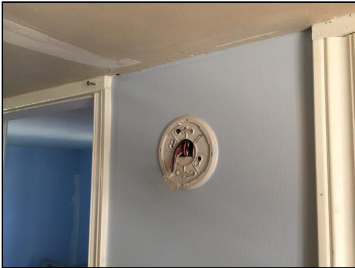
61. Removed smoke detector
