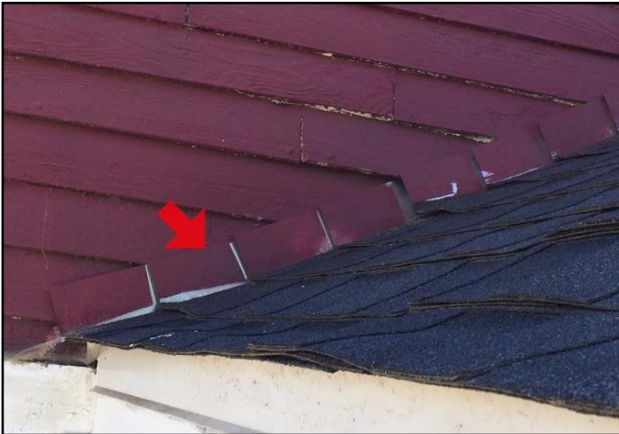
4. Flashings not properly installed
