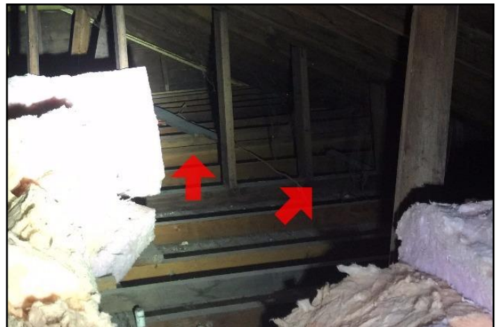
68. Gaps or voids
