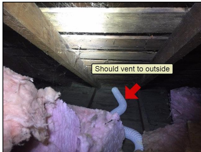
102. Bathroom Fan Exhausting into attic space
