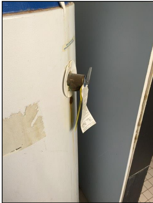
76. Discharge tube missing
