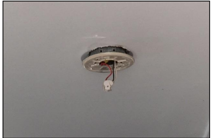
62. Removed smoke detector
