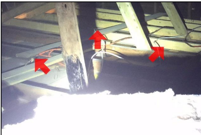
67. Gaps or voids
