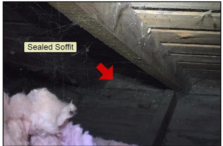
19. Missing Soffit Vents
