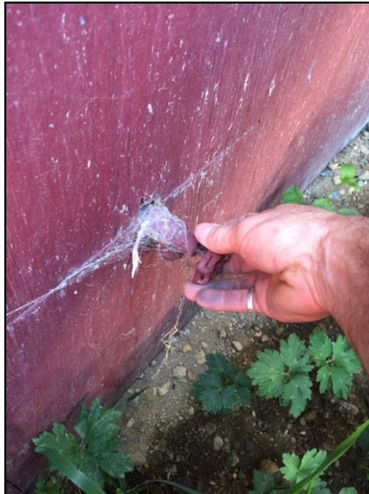
85. Hose Bib Inoperative
