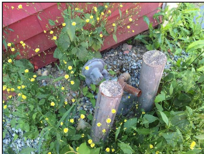
64. Abandoned Gas Service
