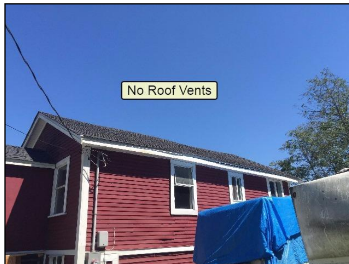
69. Missing Roof Vents
