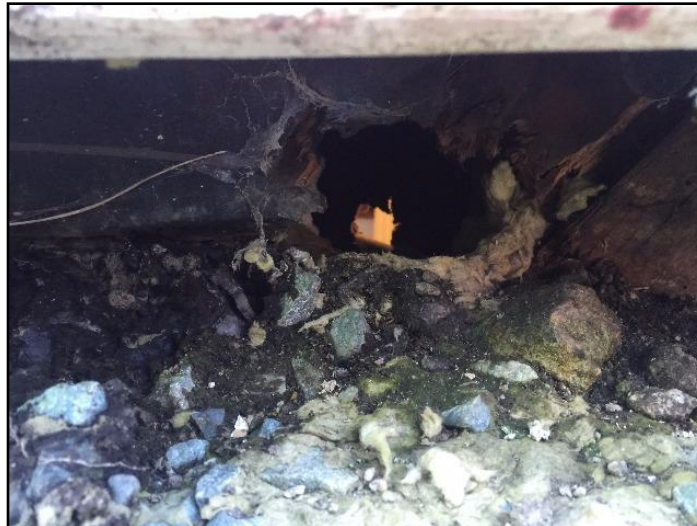
20. Rodent damage to wall
