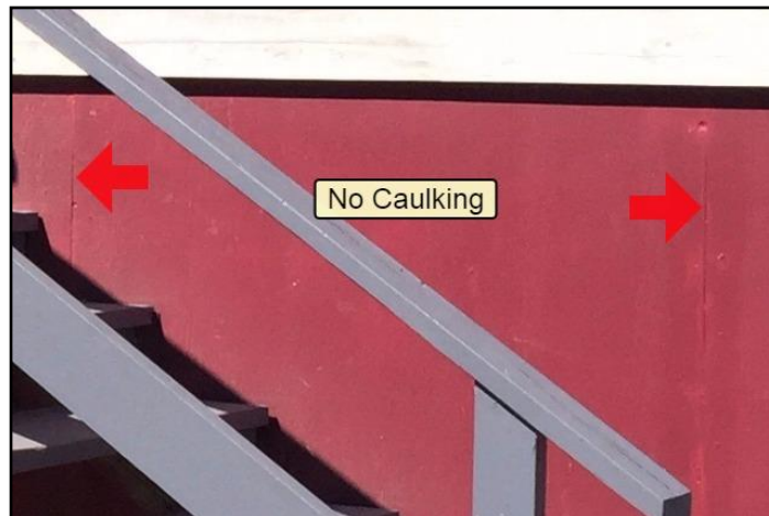
23. Missing paint or caulking
