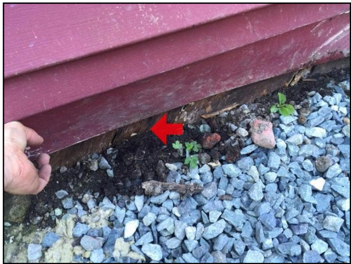
21. Too close to grade
