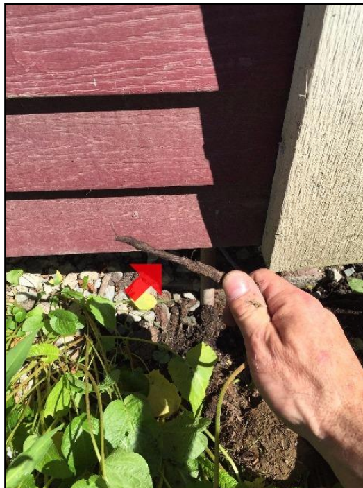
51. Ground wire corroded
