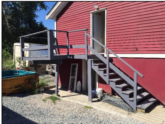
17. Unsafe Deck - Do not Use.
