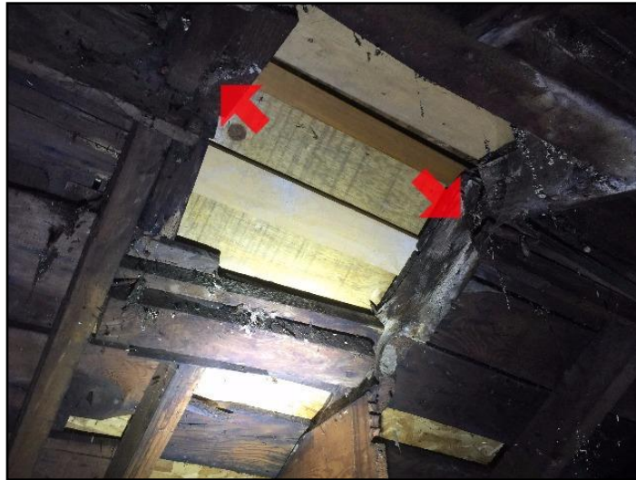
40. Rot/fire damage to roofing
