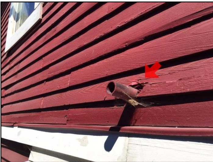
77. Abandoned Drain Pipes
