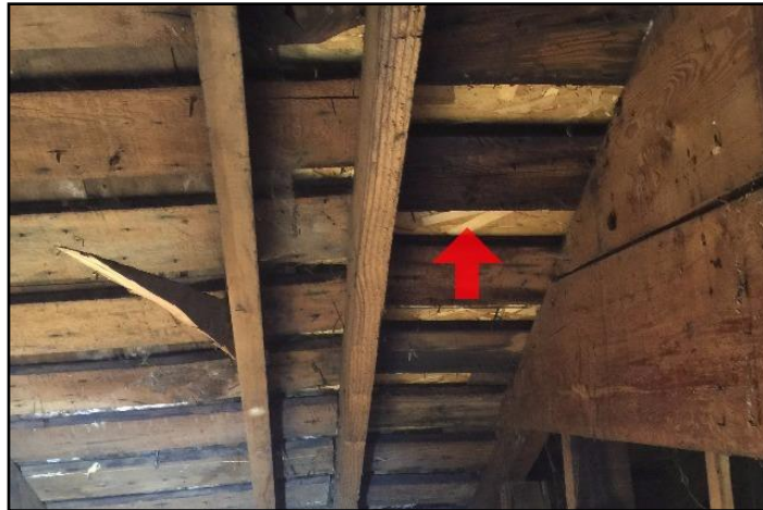
6. Patched at addition
