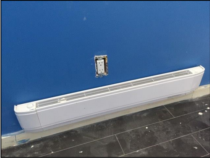
60. Above electric baseboard heaters
