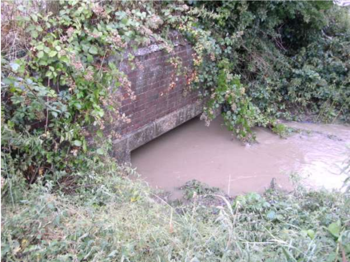
The Hastings culvert on a flood event
