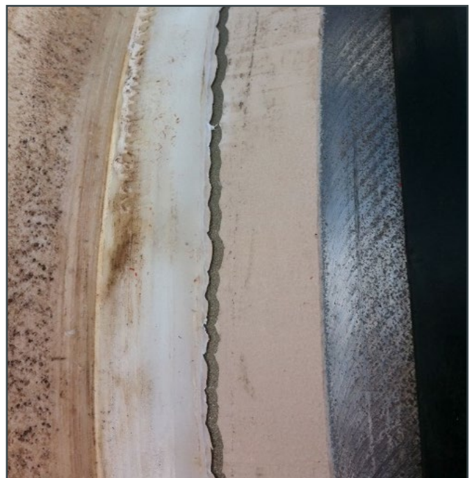
Figure 2: End Disbondment of a MLPP coating with a FBE toe (of >20 mm length vs. typically 3-5 mm)
