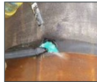
Figure 5b: Repair a localized spot of coating end disbondment on a 3LPE coated pipe using a primer + adhesive + PE melt stick
