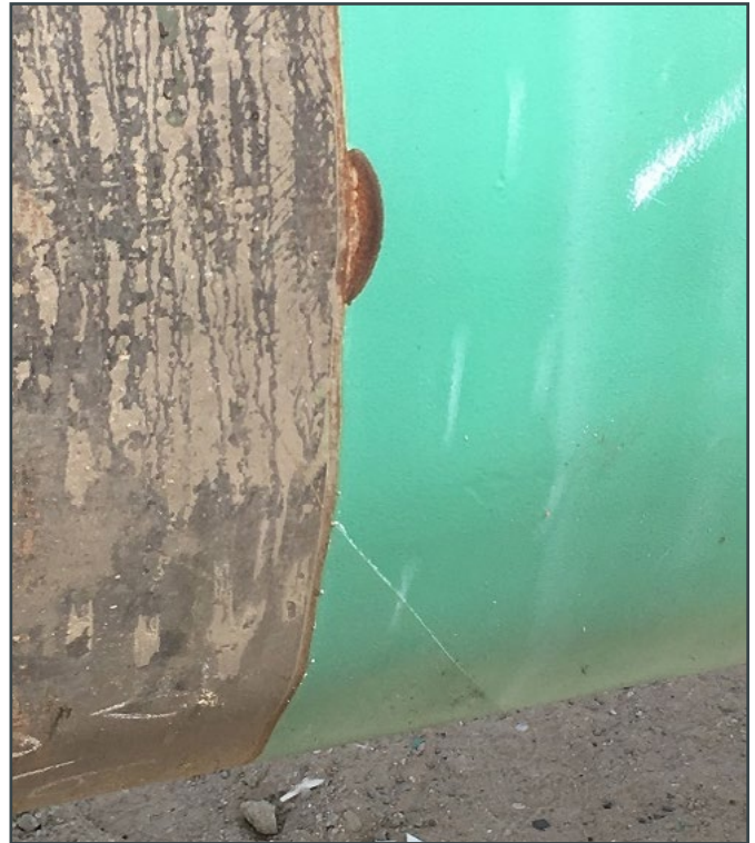
Figure 1: End Disbondment of a FBE pipe coating
