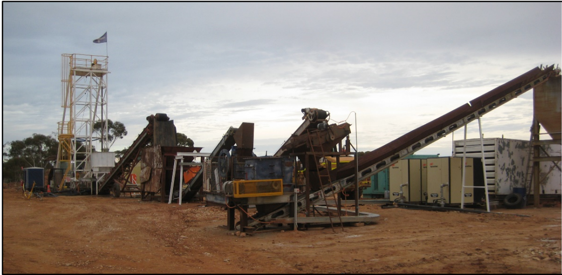
Radio crushing circuit
