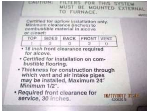
Photo X-6 Furnace Clearances Information Sticker
