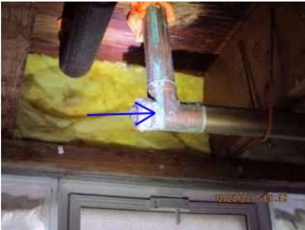
Photo X-19 Dry at the time of inspection there are signs of a long term water leak under the kitchen sink. Monitor for future leaks and any wetness.
