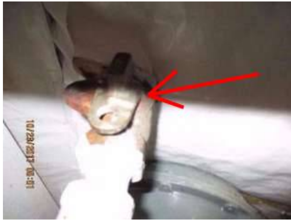
Photo X-8 Main Gas Shut off located on East side in the basement.
