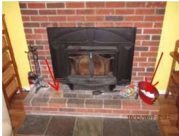
Photo X-22 With the exception of the fire glove and paper box the clearance to combustible materials is acceptable.
