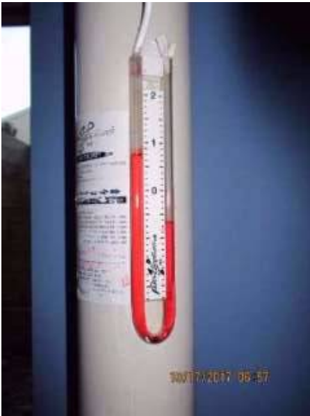
Photo X-3 Radon Mitigation system gauge in operation.
