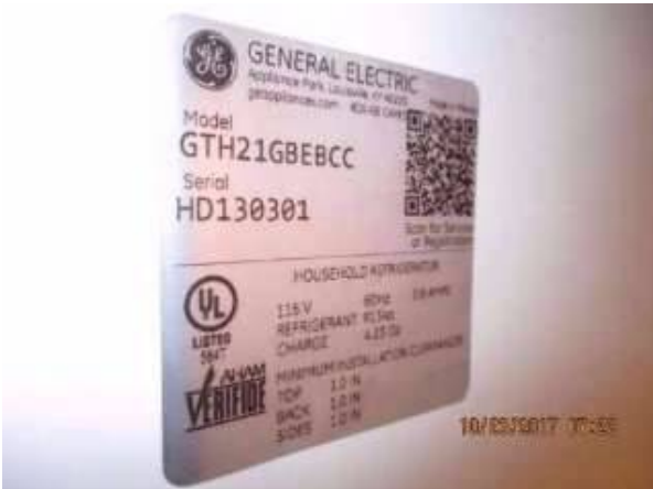
Photo 19-3 Refrigerator data plate.
