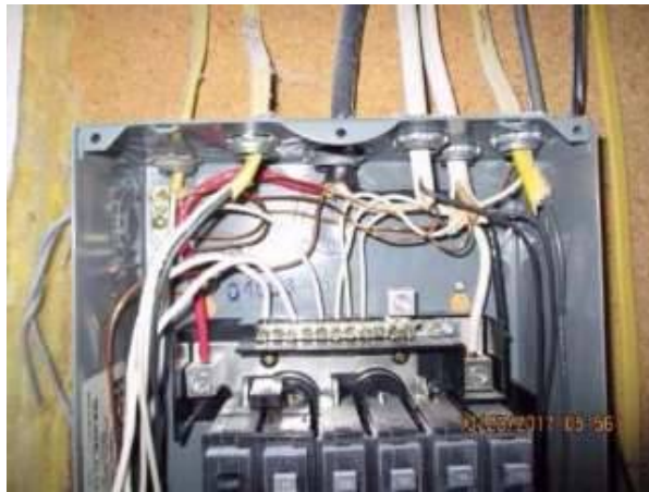
Photo X-10 Sub Panel with neutral and ground bus bars separated. GFCI's were operated except for the one breaker that was off. Breaker operates the pool and it was closed for the season. Make sure the breaker operates before you take possession of the house - talk to your realtor about the final walk through.
