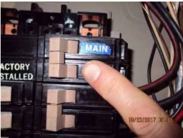
Photo 14-1 100 Amp Main Disconnect for Cutler and Hammer Principal Electric Panel
