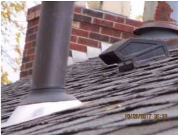
Photo 6-3 Roof penetrations appear dry at the time of inspection both inside the attic and out.
