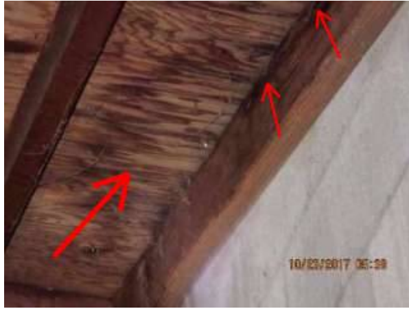
Photo 6-2 Below the chimney flashing previously pictured. Picture taken from inside the garage looking up.
