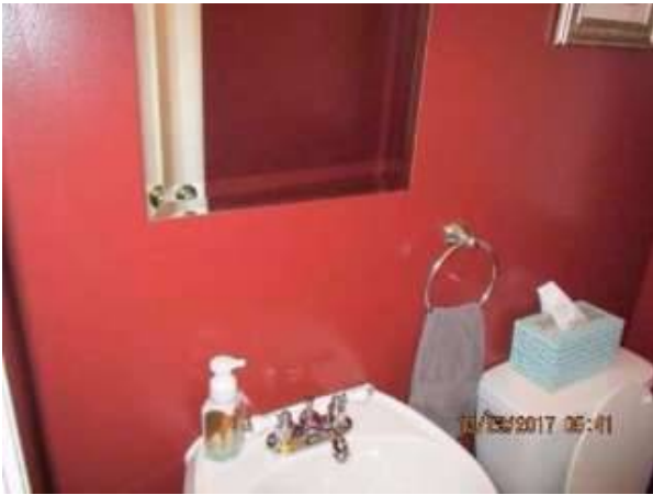
Photo X-7 No GFCI outlet in the 1/2 bath downstairs, this is an inconvenience, but could be a safety concern if someone uses an extension cord around water.
