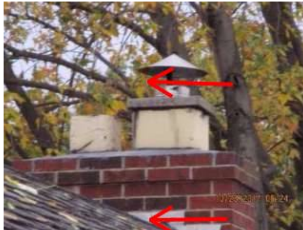
Photo X-20 Chimney height less than 3 feet above the height of the roof. At the time the chimney was made the height was probably fine. New standards today recommend 3 feet.
