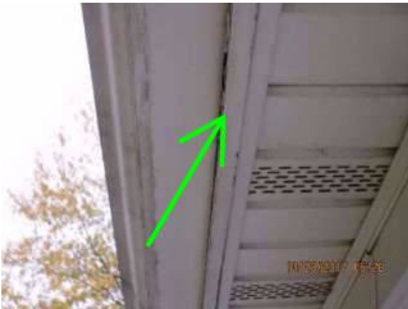
Photo X-21 Vented soffit allows for continuous airflow to the attic. Some maintenance will be needed to maintain the integrity of the fascia.
