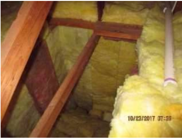
Photo X-23 Attic insulation around the stairwell has a vapor barrier and is in place.
