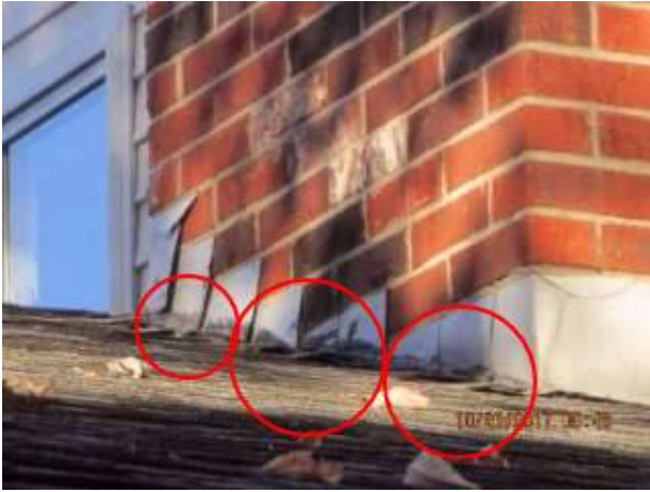
Photo 6-1 Lower roof chimney flashing is heavily caulked. No leaks at time of inspection, but visible signs of water damage from inside the garage. Check with the home owner prior to taking possession to see if the water marks were from a previous leak or repair.
