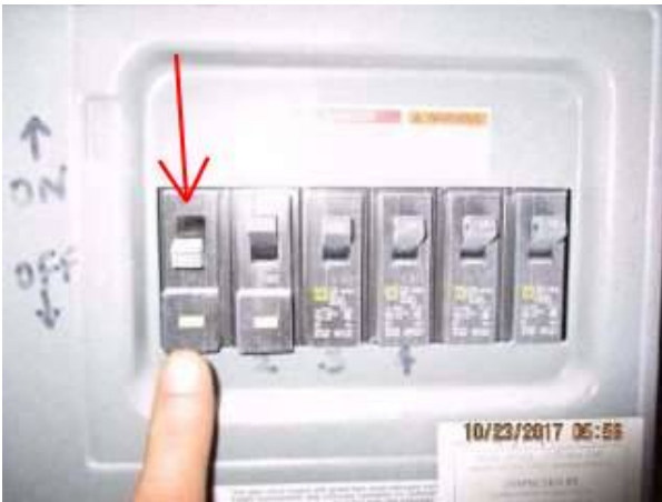
Photo X-9 This breaker was off at time of inspection and remained off during the inspection.
