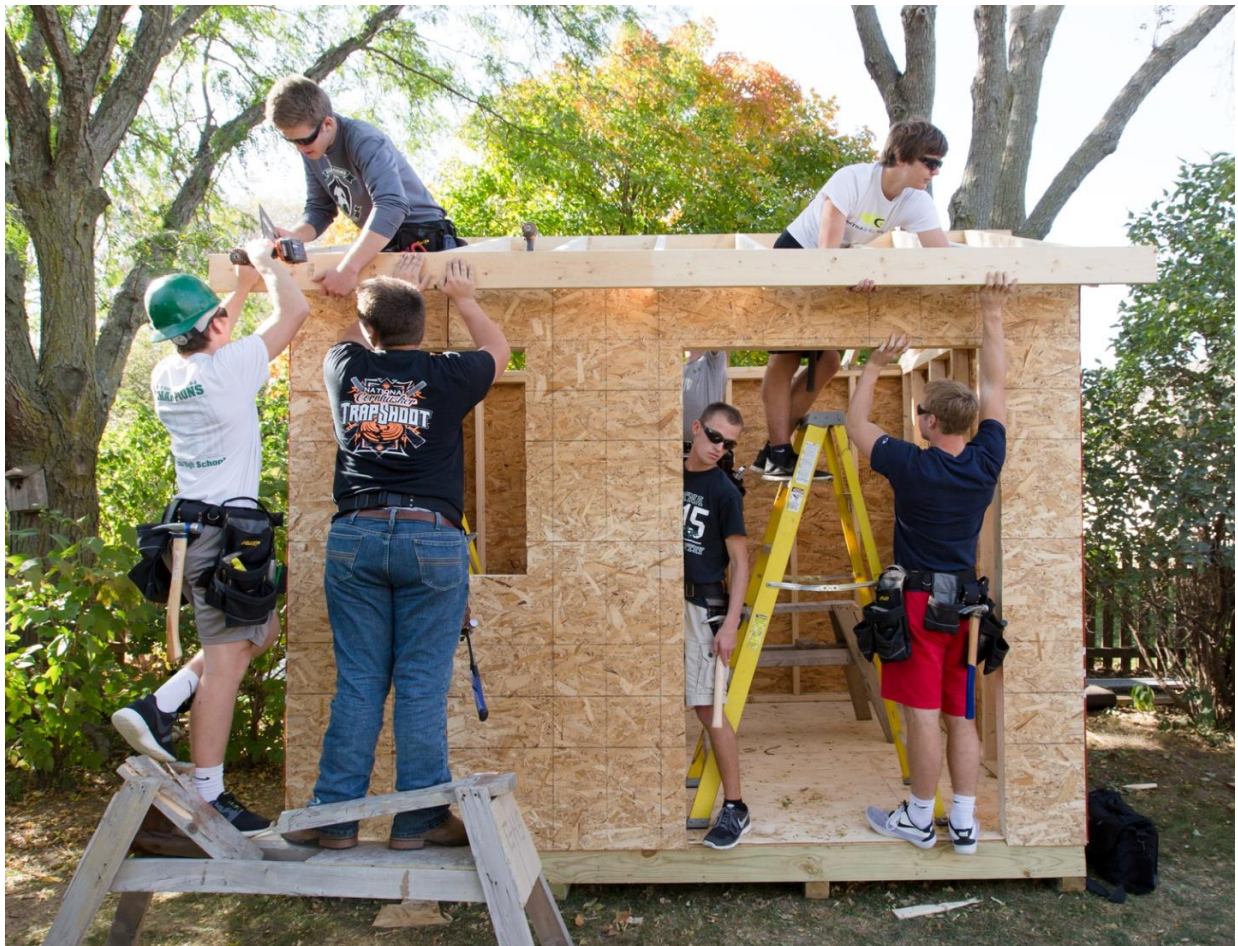
Seniors in the Gretna High School vocational building construction class construct a backyard shed as part of the Builders of the Future program, founded by Steve Skidmore with the Metro Omaha Builders Association. Working atop the shed are Jake McMahon, left, and Kyle Morbach; below them, from left, are Matt McMahon, Tyler Kudlacek, Dylan Berube and Justin Hines. KENT SIEVERS/THE WORLD-HERALD
